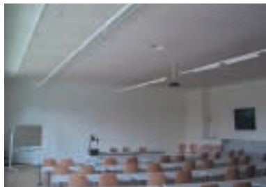
Panellings on ceiling at a schoolhouse in Seengen, Switzerland treated with SAICOS BEL AIR INDUSTRIAL COATING 7200 white
