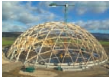
Saldome® - largest wood dome building in Switzerland - 93 m Ø, 31 m high treated with SAICOS SPECIAL WOOD OIL 0110 colourless and SAICOS HOUSE & GARDEN-COLOUR 2100 ivory
